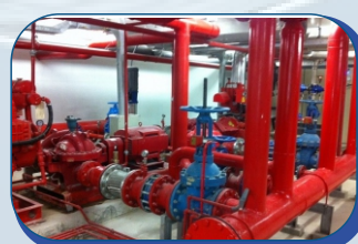
Fire Fighting Pump Room
