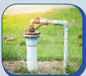
Ground Water Metering
