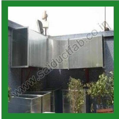
Air Conditioning Ducts
