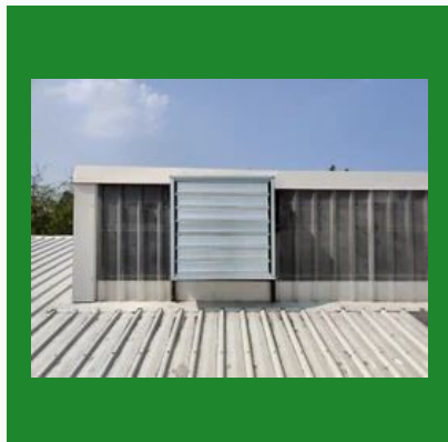
Industrial Exhaust Fresh Air Fans
