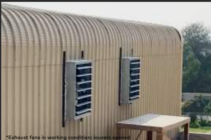
*Exhaust fans in working condition: louvers opened
