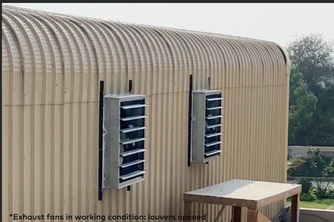
*Exhaust fans in working condition: louvers opened
