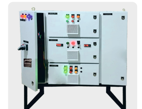
● AHU Electrical Control Panel
